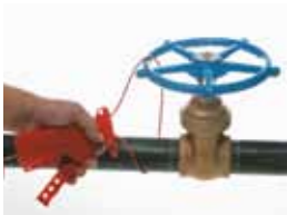
Cable lockouts - better alternative than using chain
