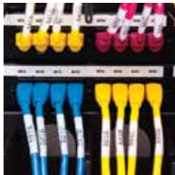
Wire & Cable Marking
